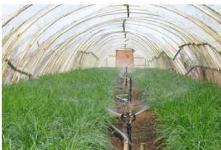
Agricultural greenhouse water supply system
